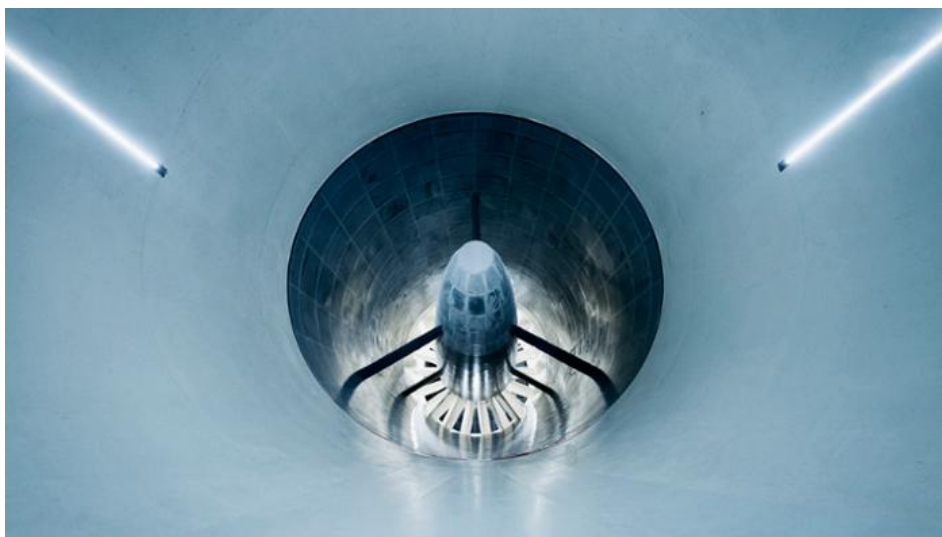
The fan's motor has an output of 7,000 kW.
